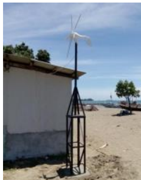
Figure 16. Bayu Power Plant. (Source: Syamsuarnis and Candra, 2020).
